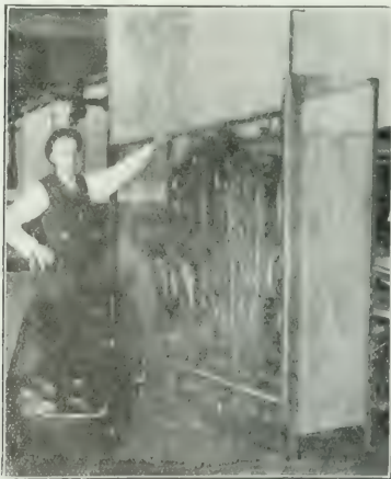
Fig. 15.—Wire-Mesh Partition Around Duplex Cutter Gears. Partition Up and Out of the Way so That Gears Are Accessible.
